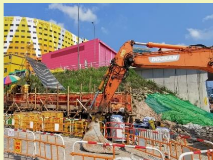
Pre-drilling works for vehicular bridges at Kai Cheng Road U-Turn Slip Road
